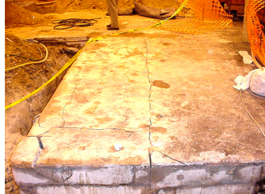
Daigh "pre-split" foundation so only half of it had to be removed.
