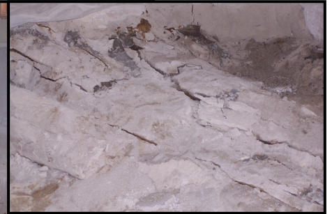
Above: Closer view of cracking
